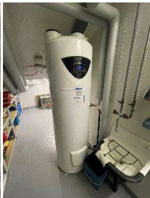
Riedmatt 1: BWW Luft/Wasser- WP
