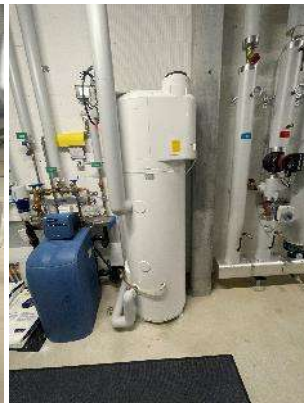
Riedmatt 3: BWW Luft/Wasser- WP
