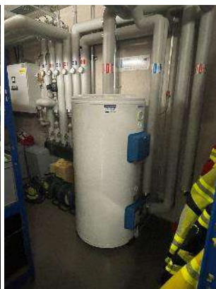
Brauchwarmwasser Luft/Wasser- WP
