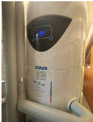
Riedmatt 2: BWW Luft/Wasser- WP
